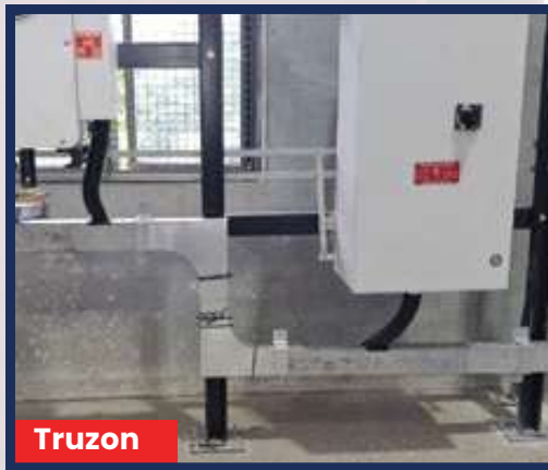
AC Cable Tray & Alignment
