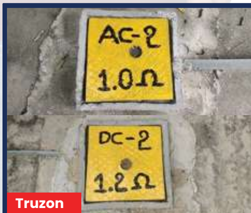
Professional Earthing with Marking
