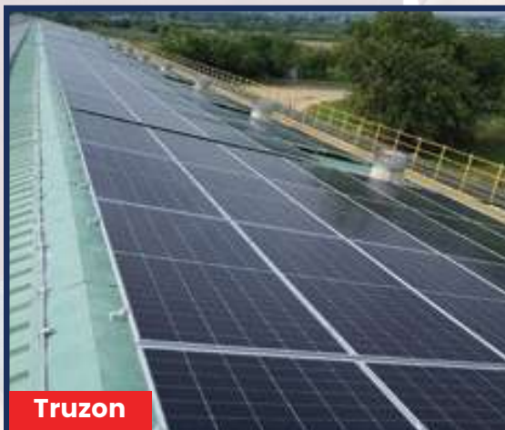
Improper Tilt Angle
